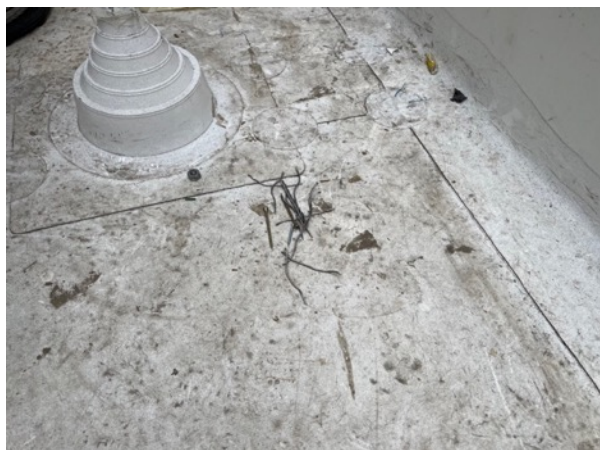
Representative Condition — Fasteners & Metal Shavings on Membrane
