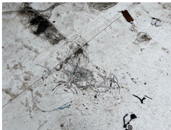
Representative Condition — Debris Present on Membrane
